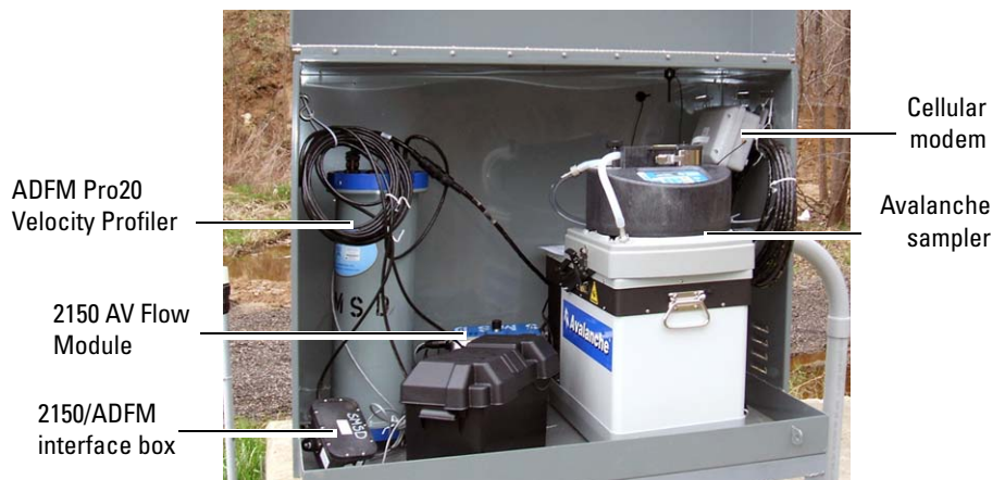
Figure 3: Avalanche sampler in environmental enclosure With cellular modem, ADFM Pro20 Velocity Profiler, and 2150 Area Velocity Module
