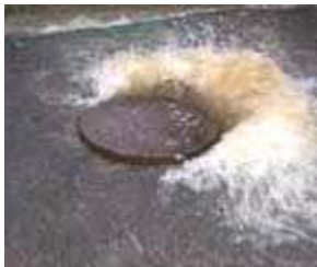
Sewer Network Flooding
