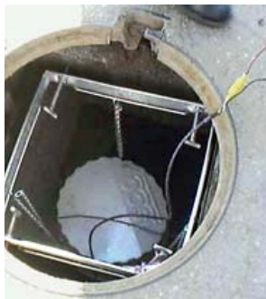
6712 Full-size sampler installation in manhole
