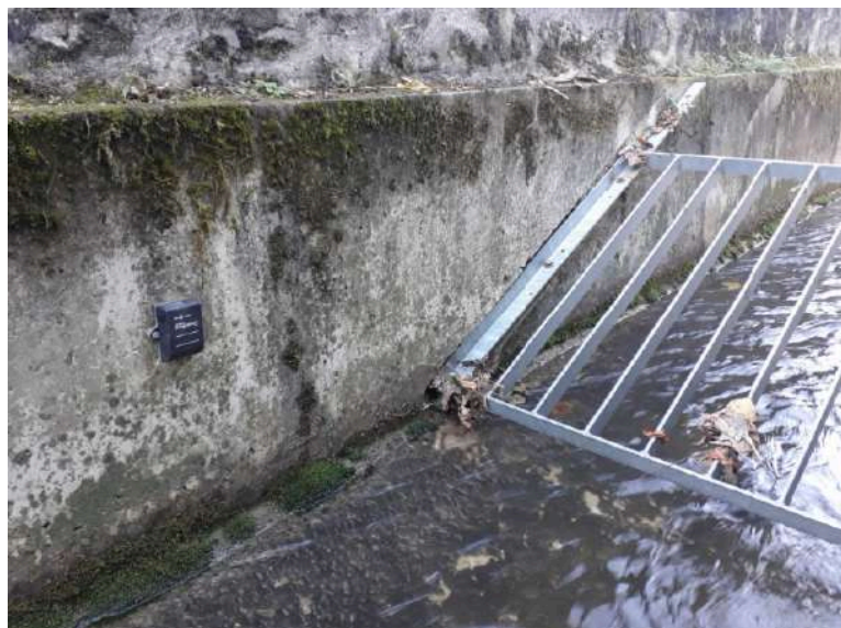
Installation for monitoring grid fouling
